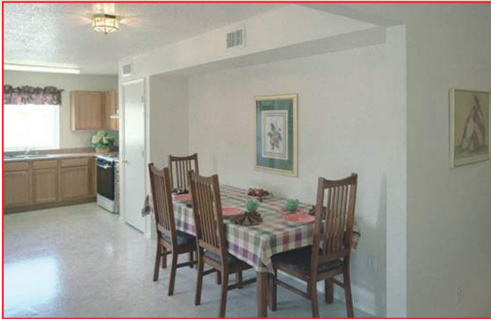
When placed in a home's conditioned space, ducts can easily blend into the décor.
