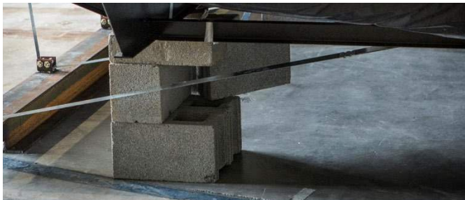
Figure 2.3. Ineligible dry-stack foundation
