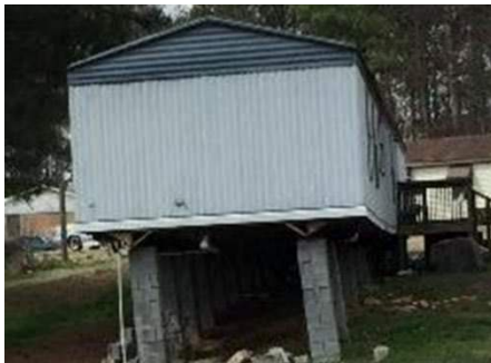
Figure 2.2. Ineligible dry-stack foundation
