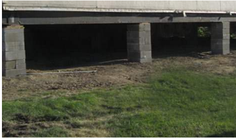
Figure 2.1. Ineligible dry-stack foundation
