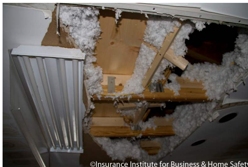
Figure 6. Photograph of collapsed ceiling in the kitchen on the unsealed roof deck side of the duplex.
